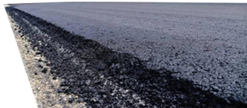
Asphalt cement retains adhesive capabilities and can be reused as a binding agent
