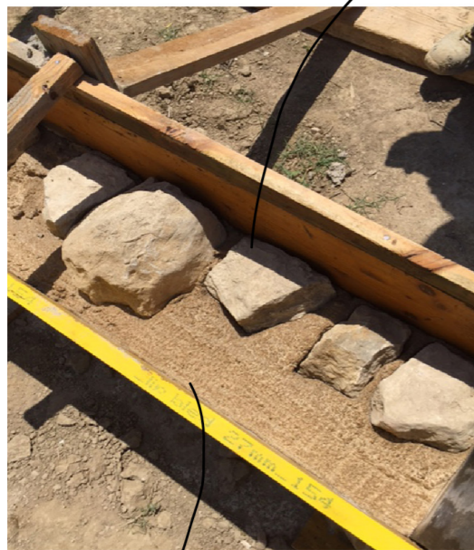
Chipped to let stone resurface (exterior side)
