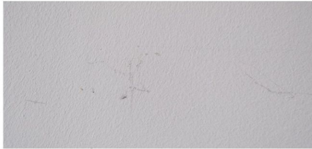
Linear stains on the west wall Unknown cause of formation
