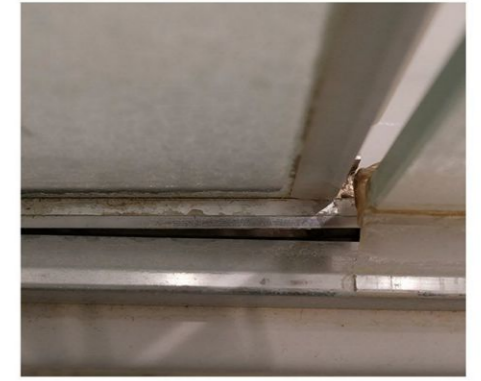
The bathroom door. Each time the door was hit hard by the other side, causing it to dent inwards
