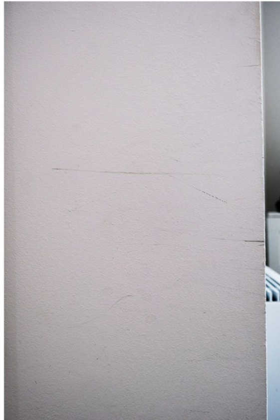
Bedroom walkway wall Scratched by boxes and large objects
