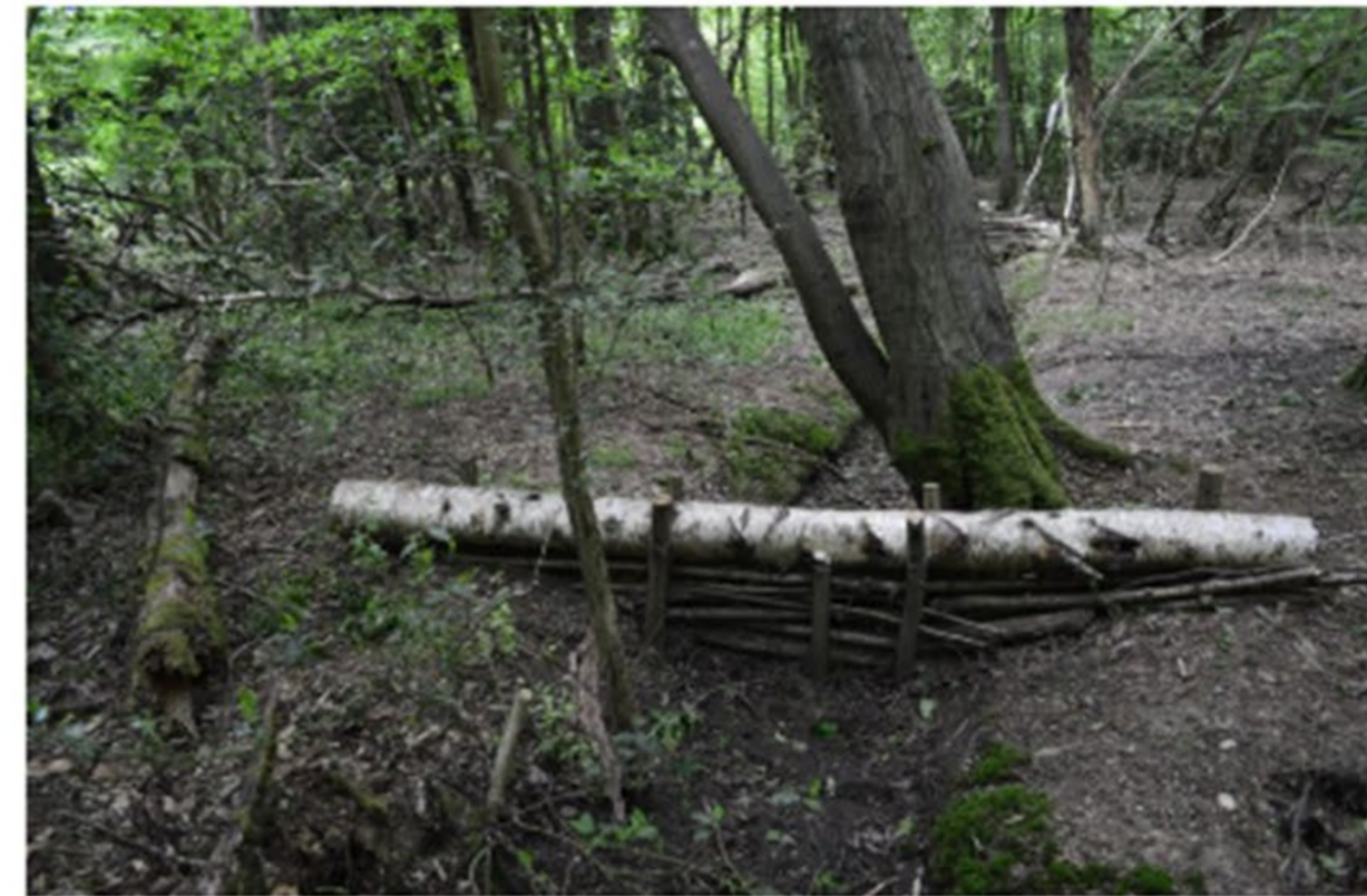
A leaky dam constructed as part of the project
